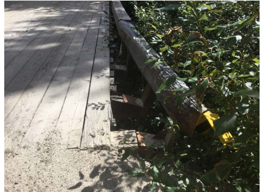
Damaged guardrail at downstream right approach
