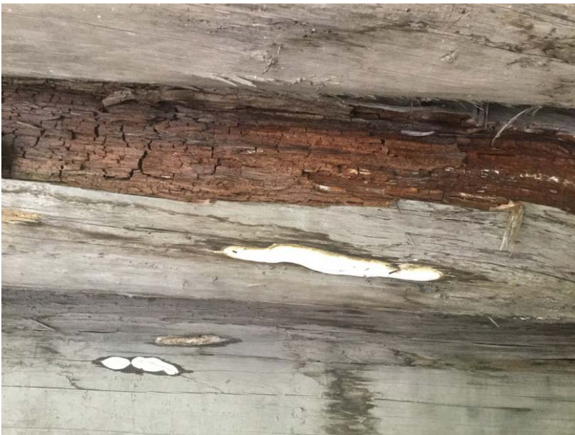
Log stringer condition
